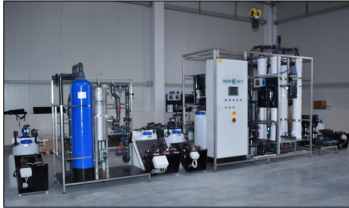
Fig. 3 The 250 m 3 /day wastewater treatment system awaiting delivery
